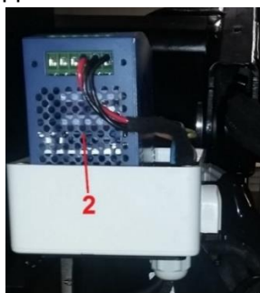
2 = omformer 230V AC/ 12V DC
